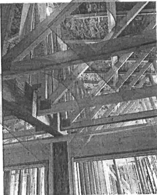
Figure 30 Building roof sheathing
